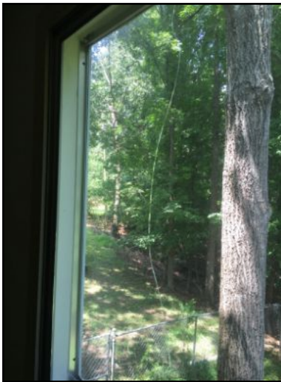
This window has crack running length of window
