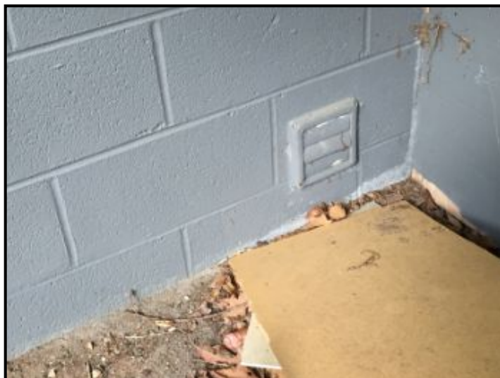
Dryer vent appears functional
