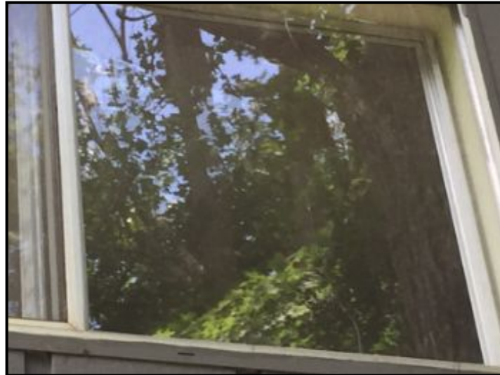
Note crack running length of this window
