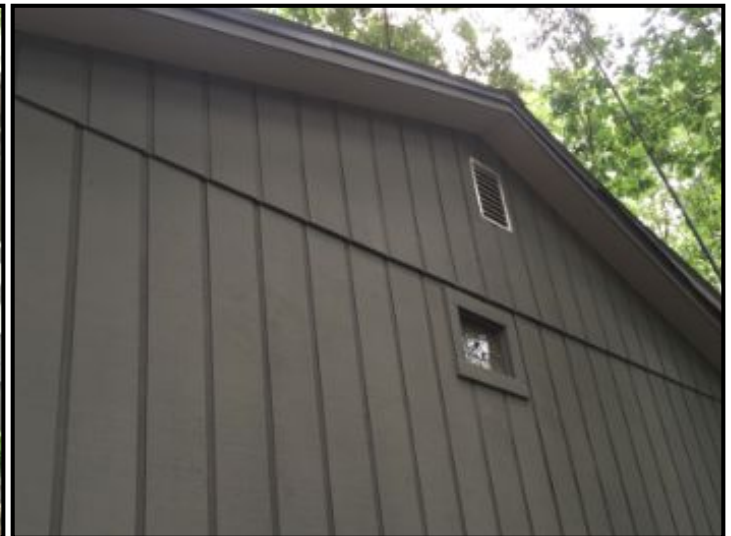
Siding looks good. Eaves and fascia board in good condition. Note gable vent in attic.
