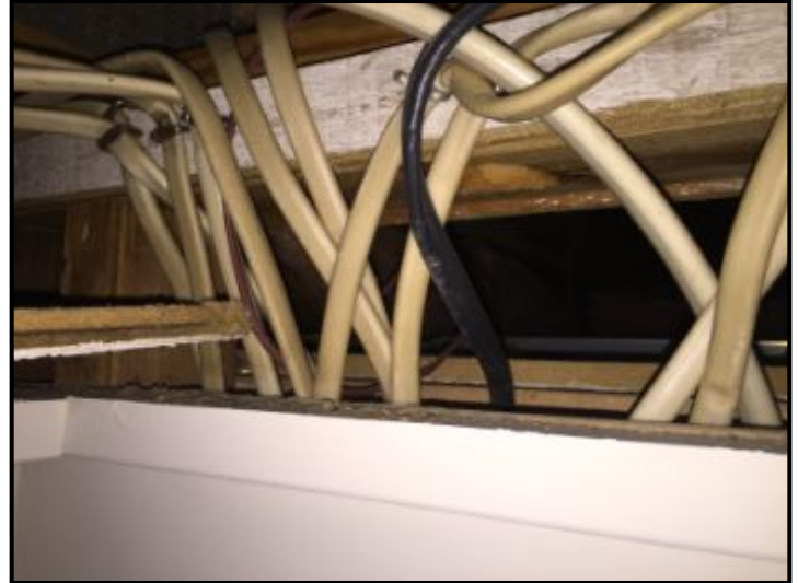
Wires above electrical panel
