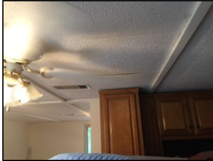
Some ceiling tiles bowing throughout house
