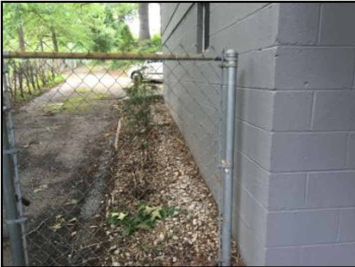
Gate looks to be in good shape. Note condition of block foundation wall.
