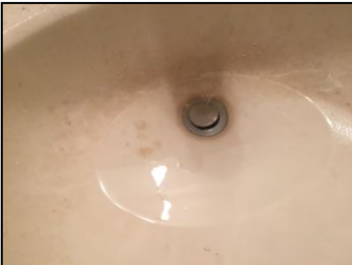
Drainage somewhat slow in downstairs sink - may need plumber to check for blockage
