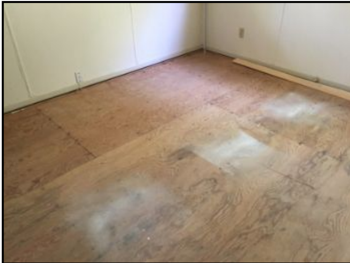
This room did not have flooring in place
