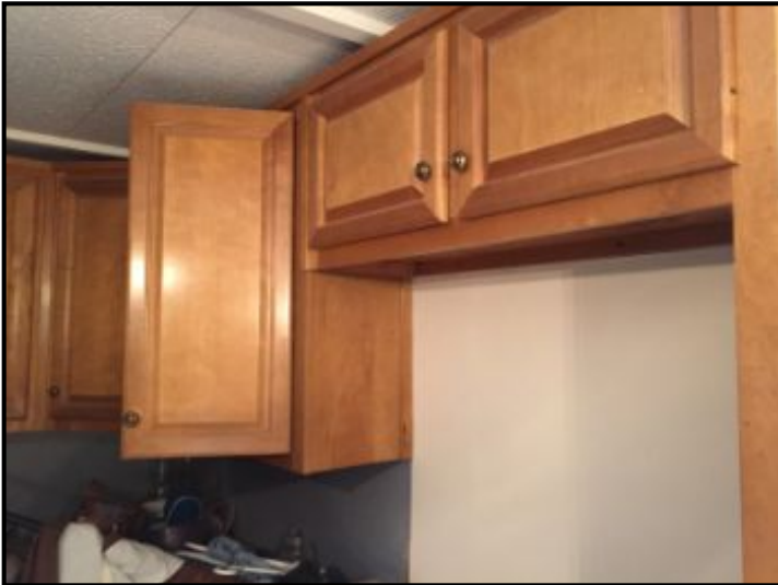
Cabinets look in good shape.
