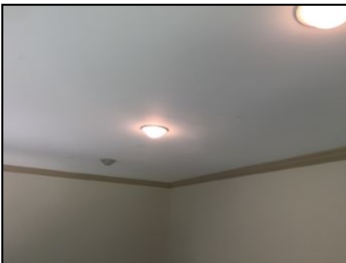
All but one light worked in this downstairs room - could be bad light bulb.
