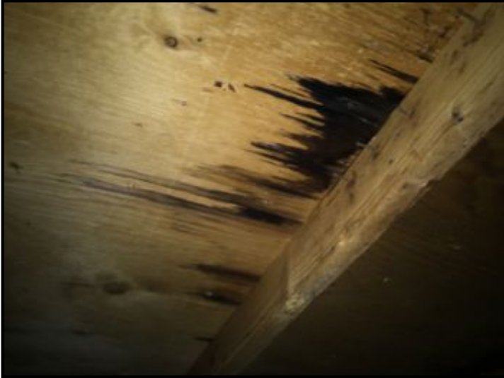
Obvious past leak noted in attic roof
