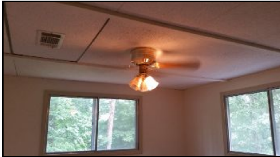
Ceiling fan and light functional
