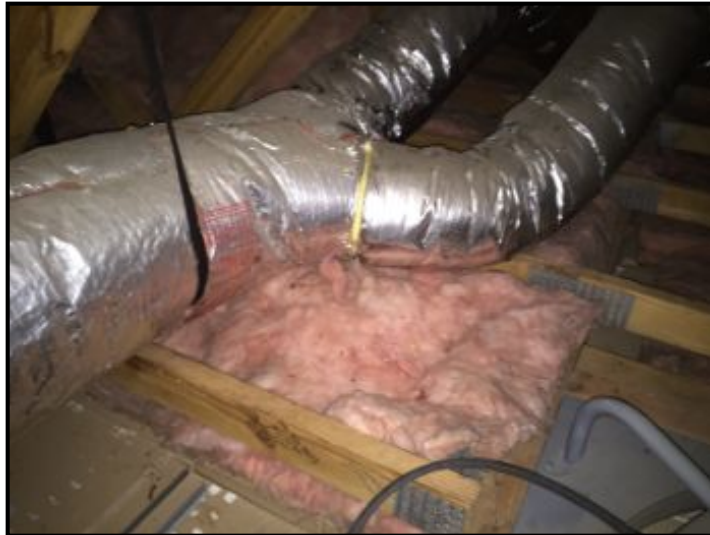
Insulation batts looked adequate during inspection - note ductwork condition
