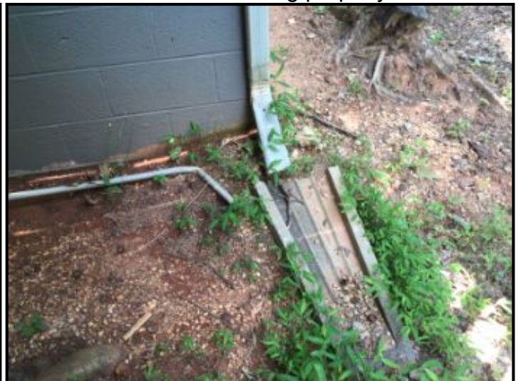
Gutter with splash block at down spout - looks to be working correctly
