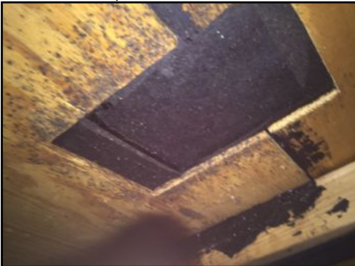
Looks to be where past leak occurred - black tar-like substance (probably Black Jack) used to seal area
