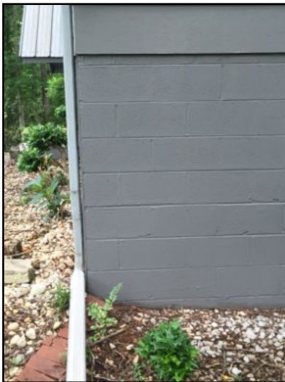
Block foundation walls look to be in good condition at time of inspection
