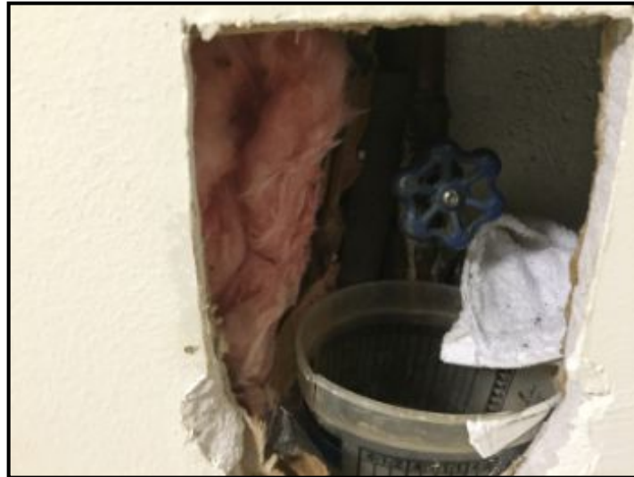
Water cut on/off located in wall of basement - My concerns are obvious past leakage and could be the source of moldy smell
