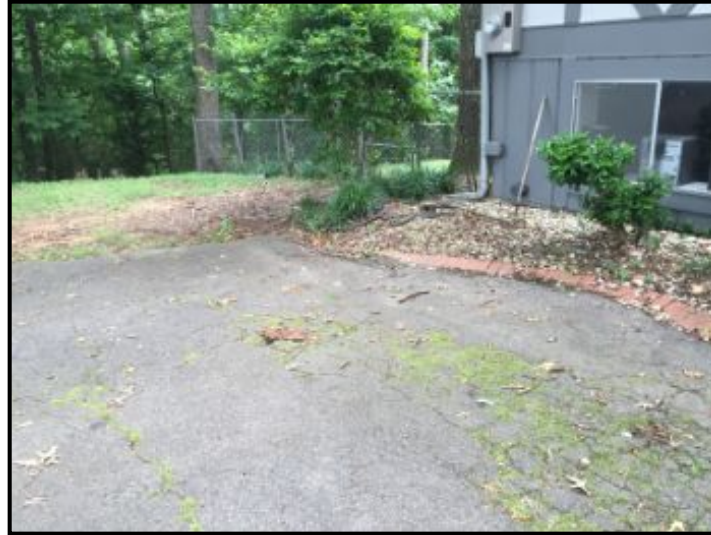
Asphalt driveway noted - normal wear for age, some cracks noted.
