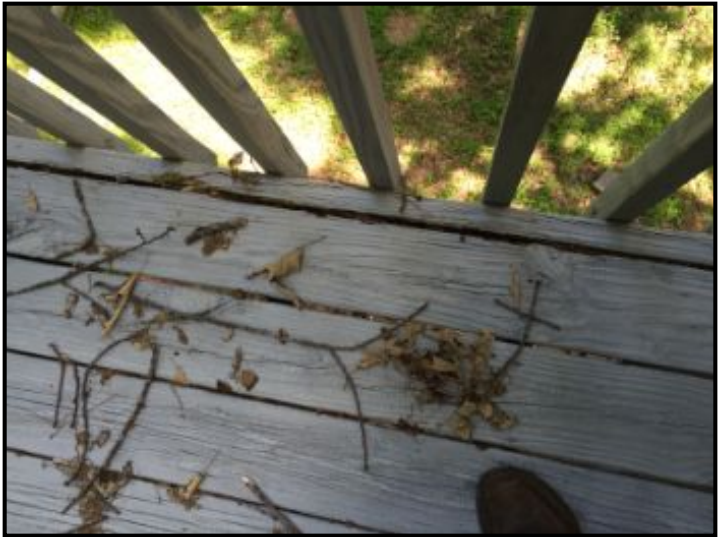
Some damage/rotting noted at edge of porch
