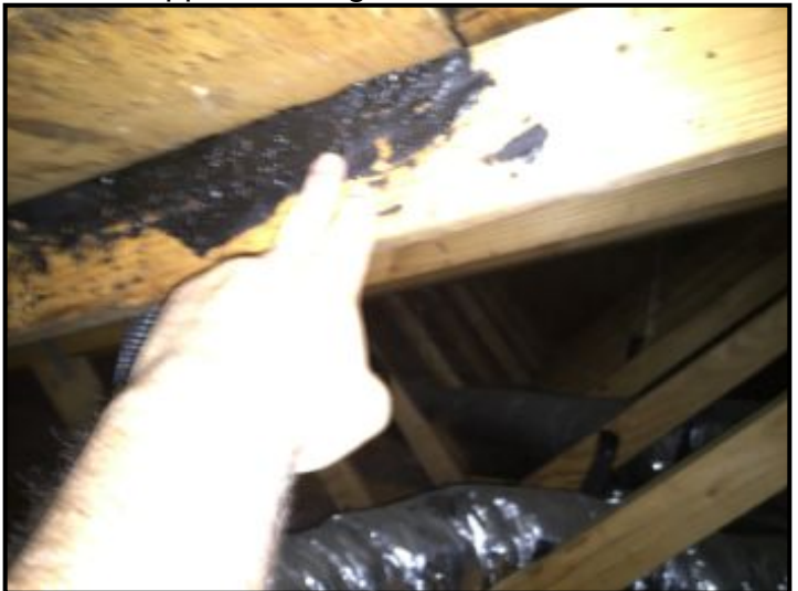
Looks like leak was sealed with Black Jack sealer
