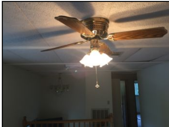
Functioned properly during inspection
