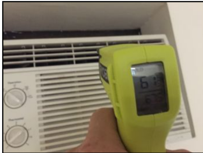
Wall unit AC working at time of inspection
