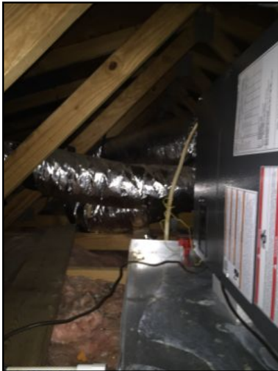
Ductwork in attic appears to be in good shape - seemed to function correctly at time of inspection
