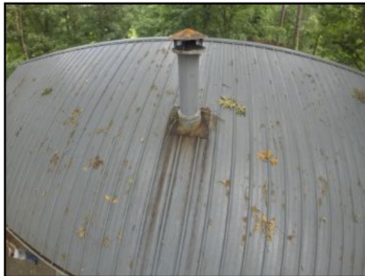
Shows sign of rust and some degradation around boot - consider replacing in the future
