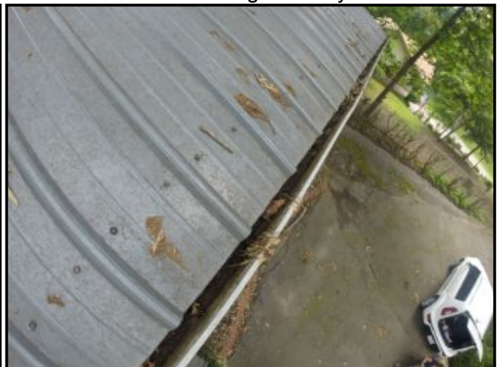
Gutters need cleaning
