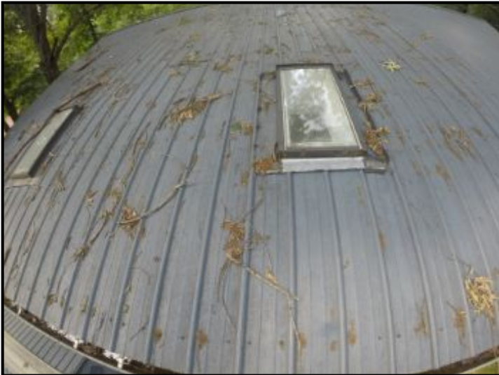
Sky Lights look good and properly installed from what I see - flashing in place
