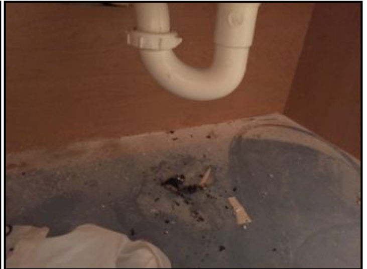
Possible past leakage or just dirty, no leaks noted at time of inspection
