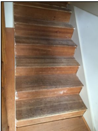
Functioned during inspection
