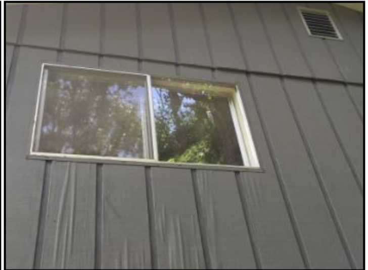
Siding beneath windows showing some swelling - should have this checked when replacing windows - make sure seals are properly installed when new windows are in place.
