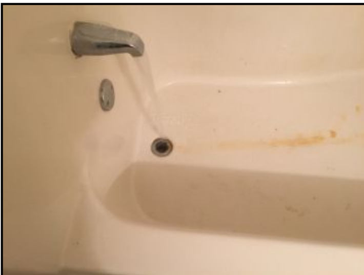
Tubs worked at time of inspection
