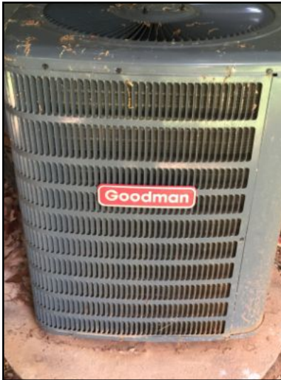
Goodman Heat pump functioning correctly at time of inspection
