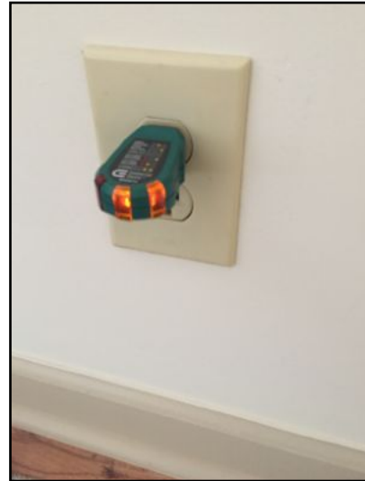
All outlets checked seem to be working properly
