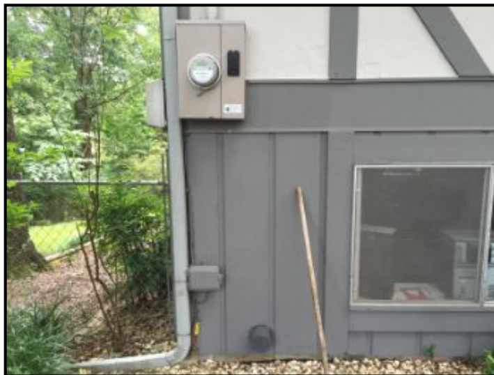
Power main location at front of house. Also phone service. Downspouts look to be in good condition and functional. Siding also appears to be in good shape.
