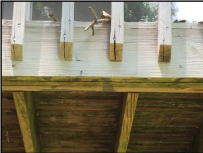
Railing has cracks where nails are used to attach to the porch - recommend replacing with new wooden rails
