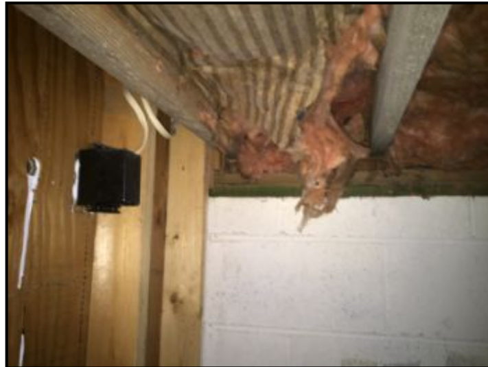
Underneath stairs some insulation batts need fixing/replacement
