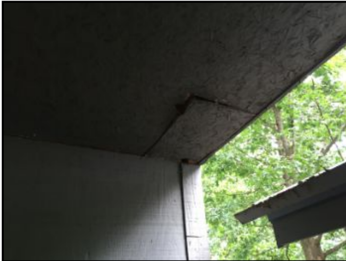
Siding looks good - someone cut an access area in bottom flooring probably to access/run electrical cable - I did not verify function.
