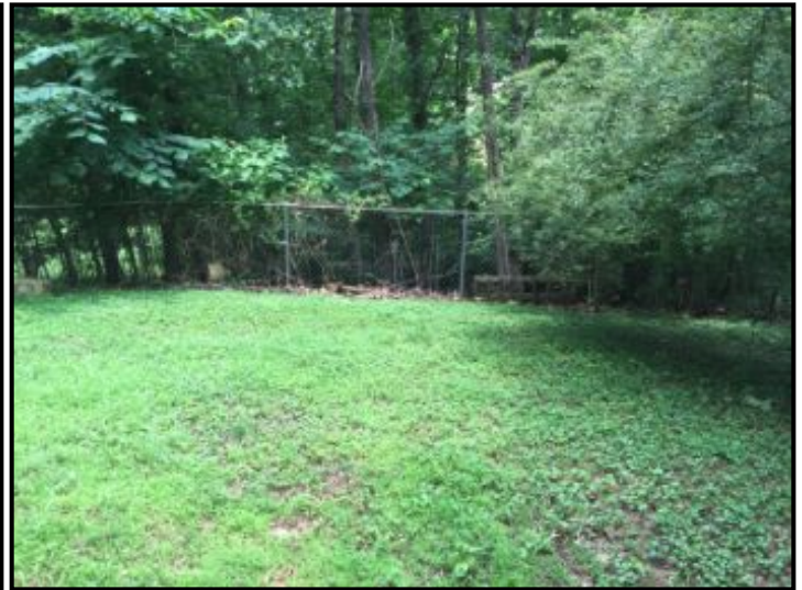
Grading appears to slope away from the house - no sign of problems with drainage.
