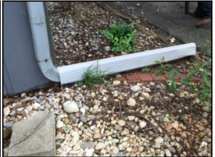
Gutter drainage is away from the house - appear to be functioning properly
