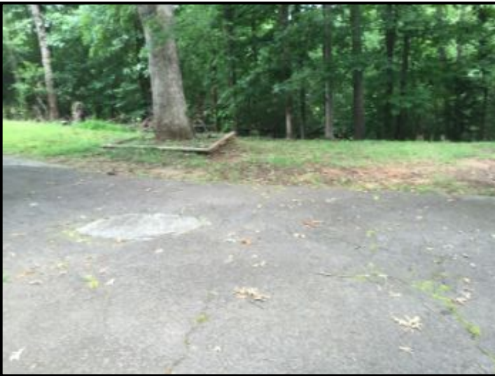
Grading appears to slope away from the house
