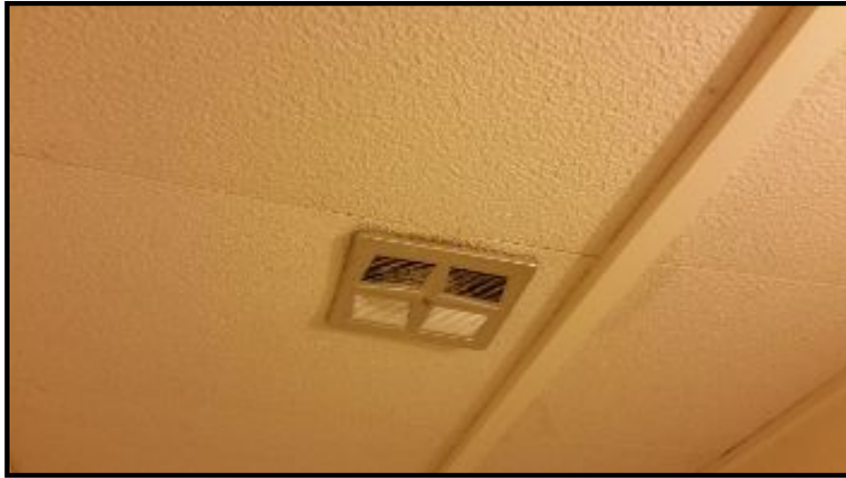
Exhaust fan working at time of inspection
