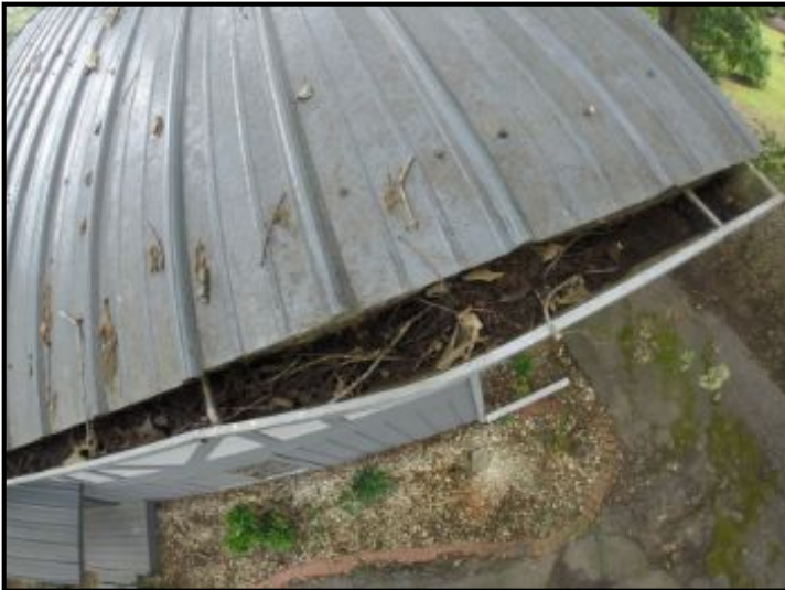
another pic of debris in gutter
