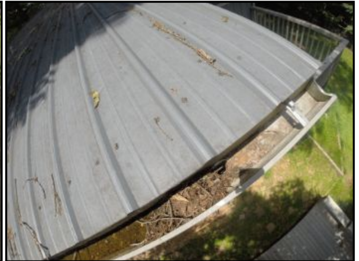
Gutter drain almost clogged because of debris
