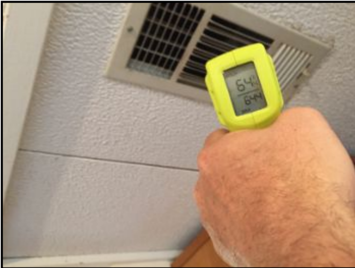
AC vents working at time of inspection
