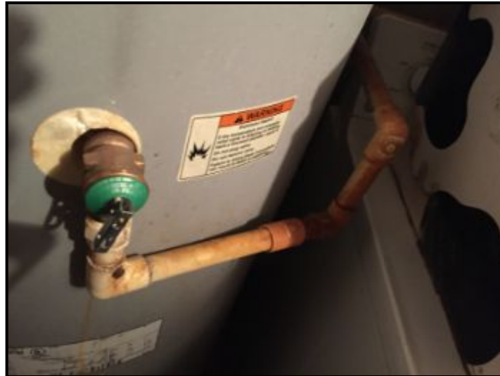
Water presure relief valve - shows some signs of past leakage.
