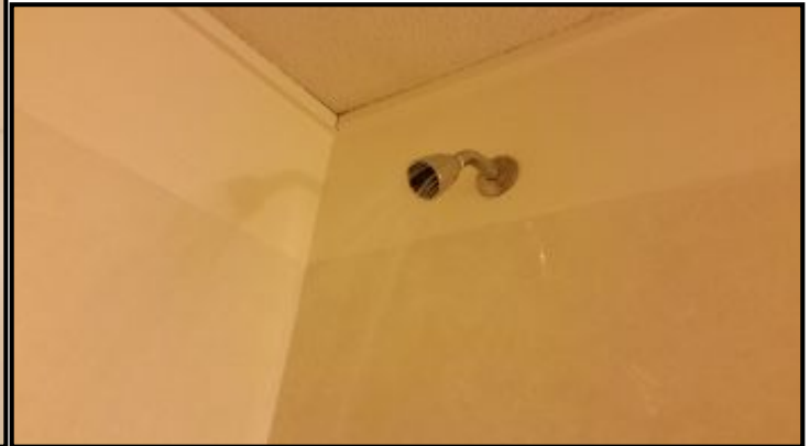
Shower functioning at time of inspection
