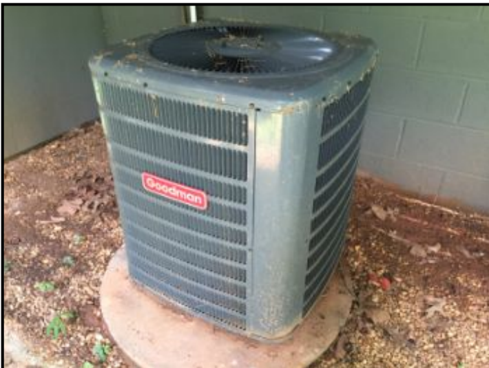
Heat pump functional at time of inspection - looks to be in good condition - looks fairly new.
