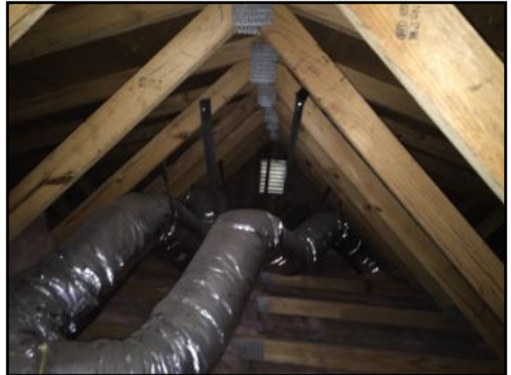
Ductwork looks to be in good shape in attic - note support beams in good shape and anchored with metal gusset plates.
