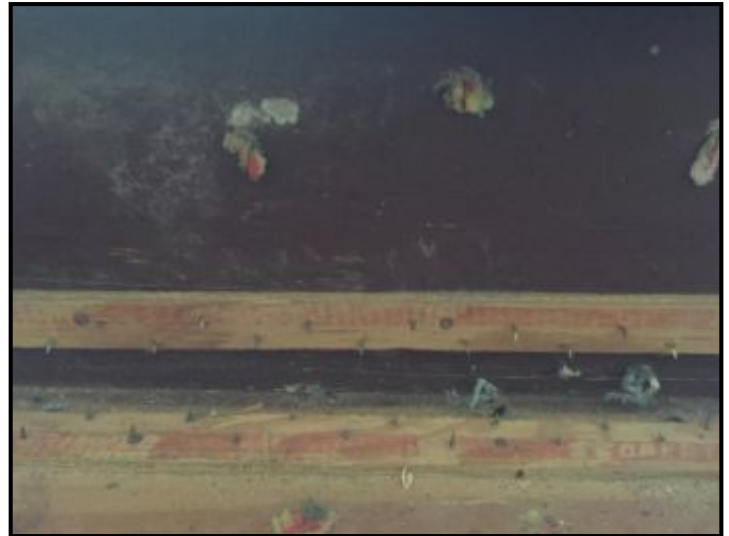
Stairs leading up from basement - obvious where carpet was removed exposing small nail strip
