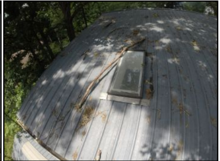
Sky Light looks good - remove debris from roof
