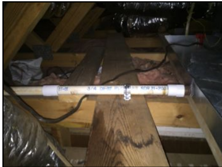
Water pan connected to PVC drain pipe
